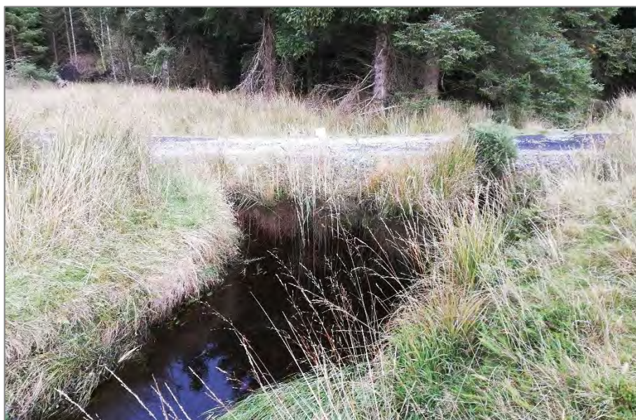
Plate 7-9 Site OHL2A – existing (collapsed) culvert viewed upstream with drained stream flowing to Lough Atorick in foreground
